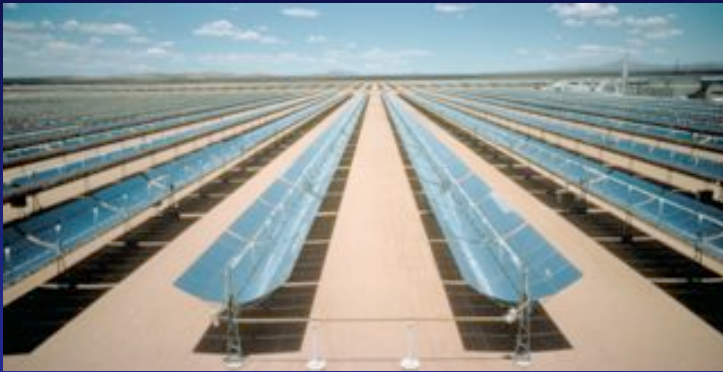
Concentrated solar-thermal, 2-axis tracking (90 MW, CA)
